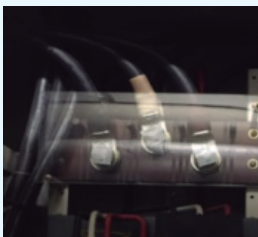
An abnormal exothermic of wiring
